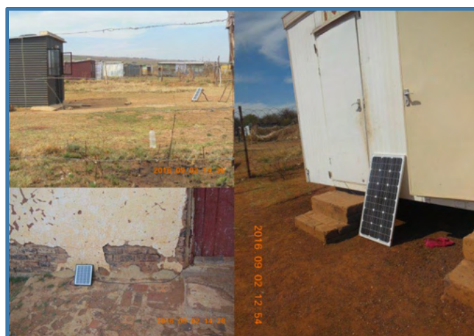
Figure 4.29 Solar panels in Thusanang (Equispectives, 2016).
