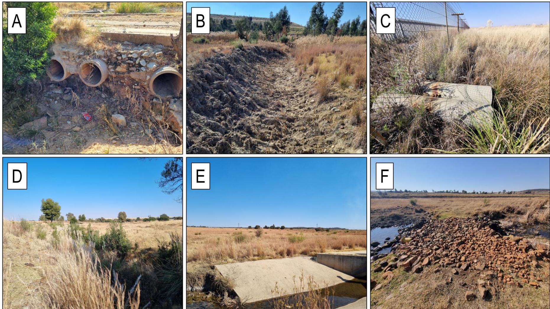
Figure 4-2: Some of the impacts observed during the 2025 survey, A) geomorphological modifications due to road crossings, B) invasive Eucalyptus sp. proliferation and trenching, C) additional water inputs, D) Acacia sp. encroachment, E) channel, bed and flow modification, F) channel, bed and flow modification due to rock dumping for crossings.
