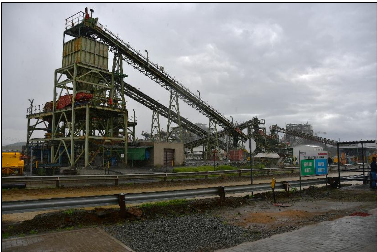
Figure 4: Voyager Crushing Plant
