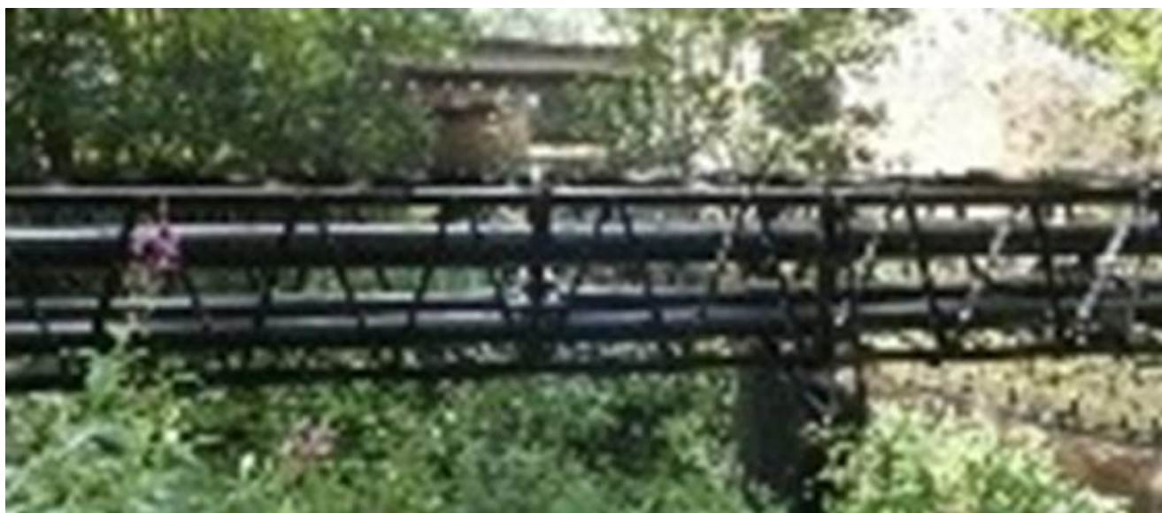
Figure 37: Typical Pipeline Gantry
